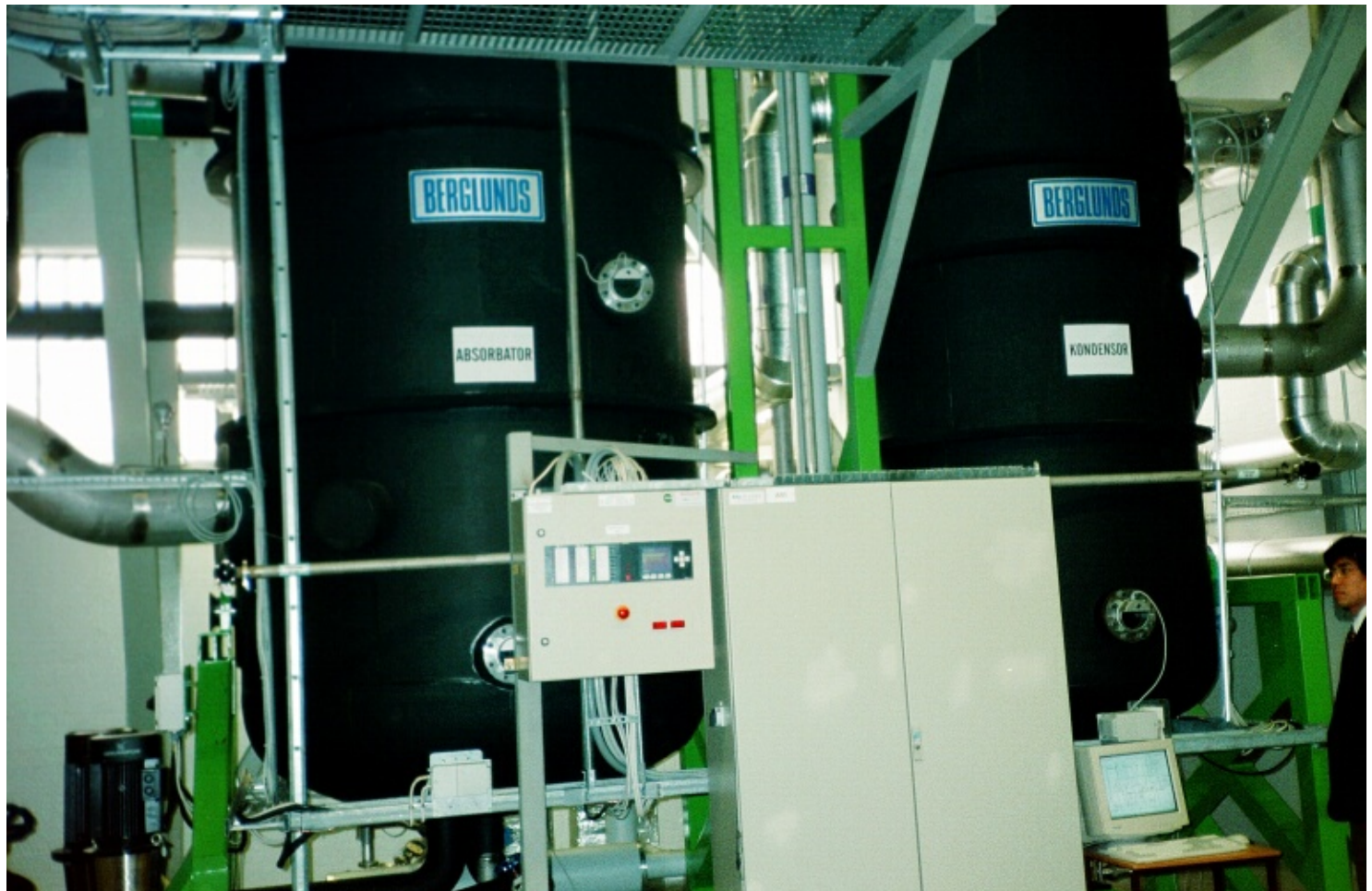
Low temperature driven absorption chiller with falling film heat exchangers Demonstration plant with 1 MW cooling capacity in Gothenbourg
